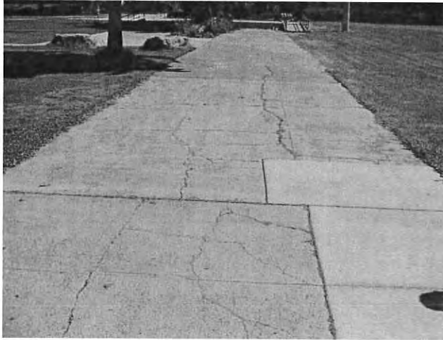
Paving Showing Stress
