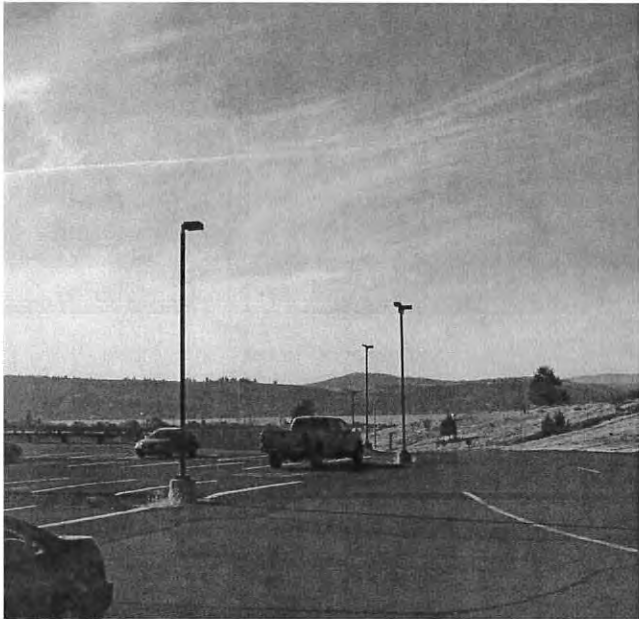
New High Mast Lights at Cornett West Lot
