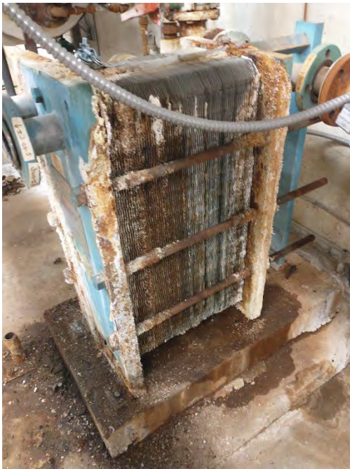
Figure 2 - Owens Hall heat exchanger, beyond useful life, from incident on September 14, 2022
