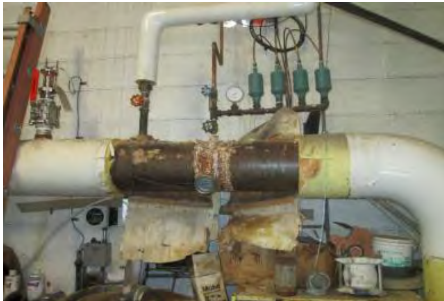
Figure 4 - Geothermal Mechanical Building; existing piping has been in service for 60 years.
