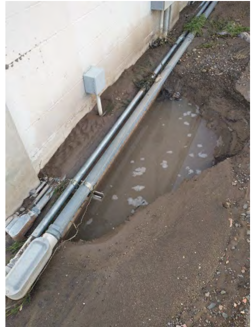
Figure 1 - Main pipe from Well #6 ruptured at building foundation footing, from incident on September 7, 2022
