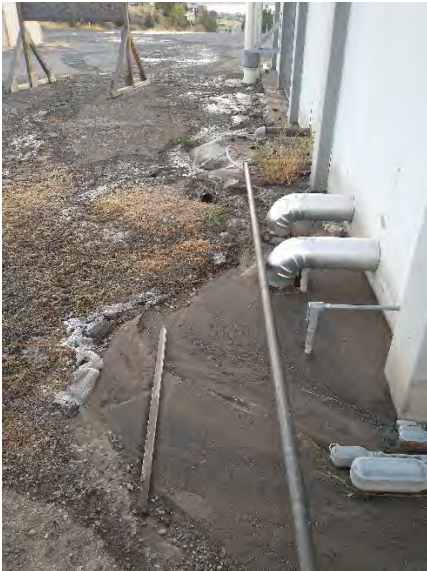
Figure 2 – Well #6 main pipe rupture flooding, from incident on September 7, 2022
