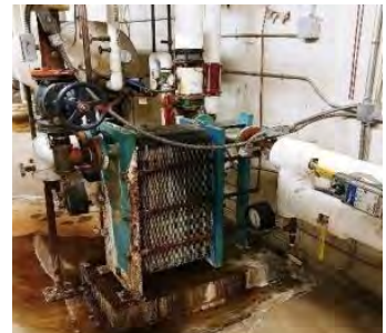
Figure 11 - Heat Exchanger; leaking a safety hazard, needing repair/replacement based on respective building
