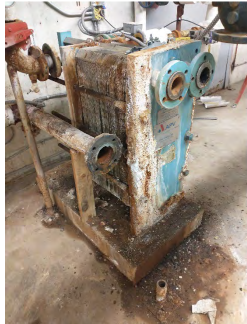
Figure 1 - Owens Hall heat exchanger, beyond useful life, from incident on September 14, 2022
