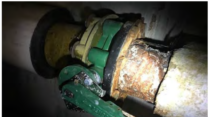
Figure 3 - Ruptured pipe, from incident on June 14, 2022
