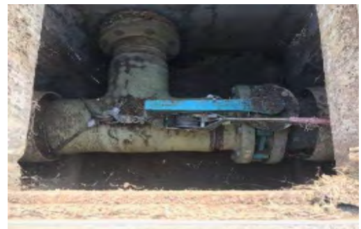
Figure 10 - Geothermal supply piping; valve inoperative, pipes questionable
