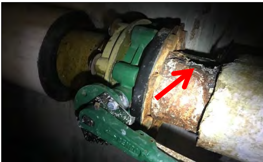
FIGURE 4: RUPTURED PIPE IN TUNNEL
