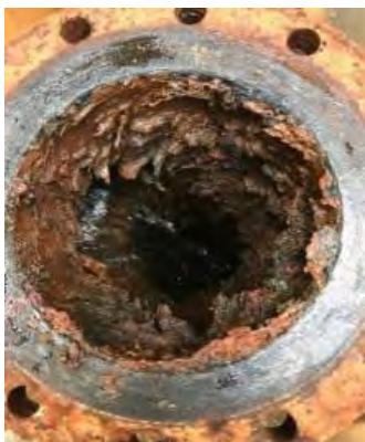
Figure 7 - Well #1 in need of cleaning and repairs
