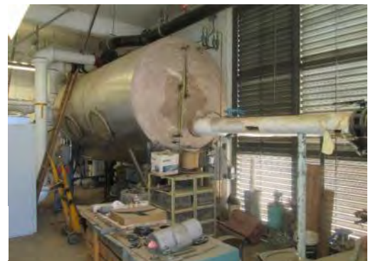
Figure 9 - Existing storage tank corroded and at risk of failure
