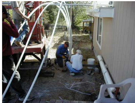
New Downhole Heat Exchanger (DHE)
