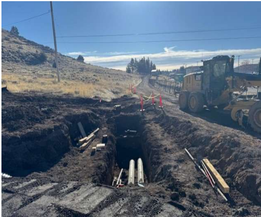
Well 5 with New Supply & Return Pipe
