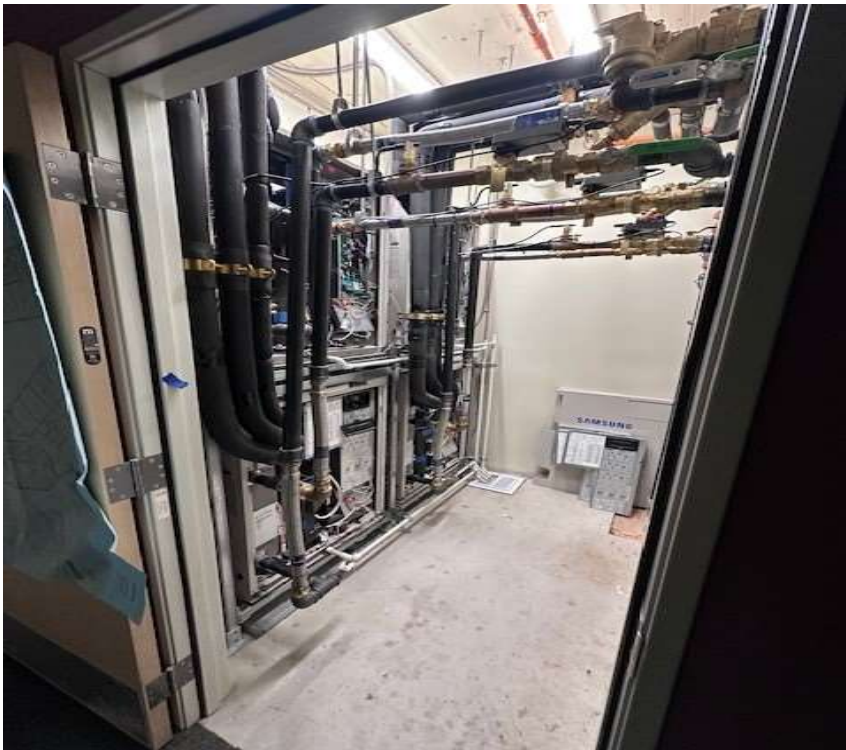
Typical Building Heating & Cooling Mechanical Room
